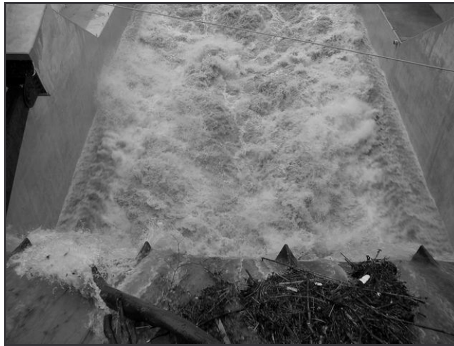
Fig. 6. Example of stable stilling basin working at Vrhovo HPP spillway (1 st spillway equipped with the side dissipation beams)
