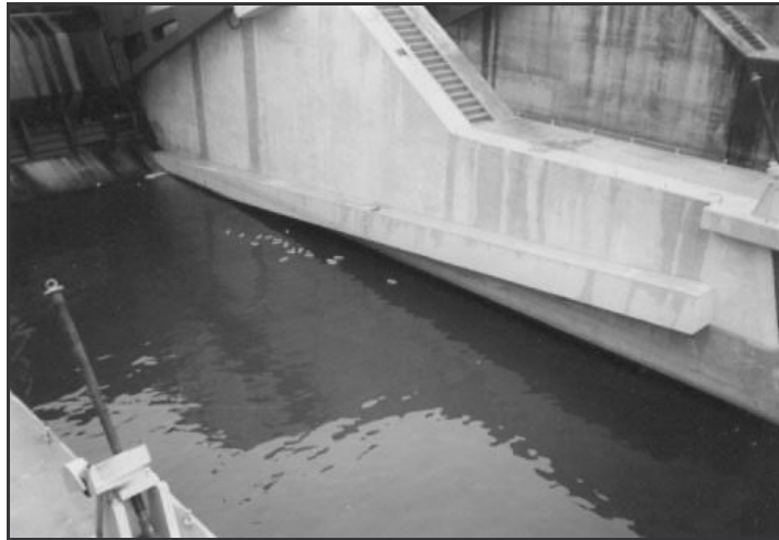
Fig. 3. Side dissipation beams in the 1 st stilling basin of the Vrhovo HPP dam
